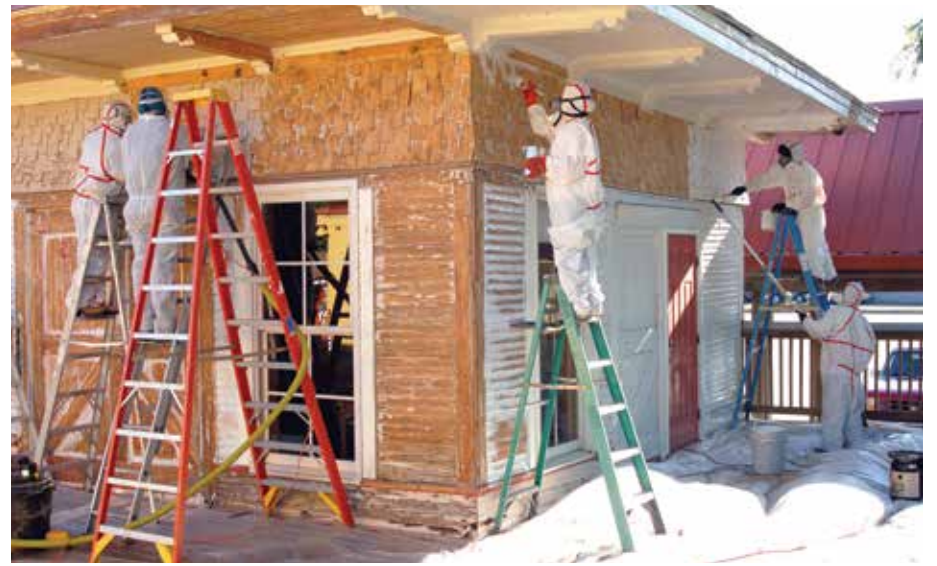
The Depot is getting renewed with a fresh coat of paint, and will become the office of the city inspector.
